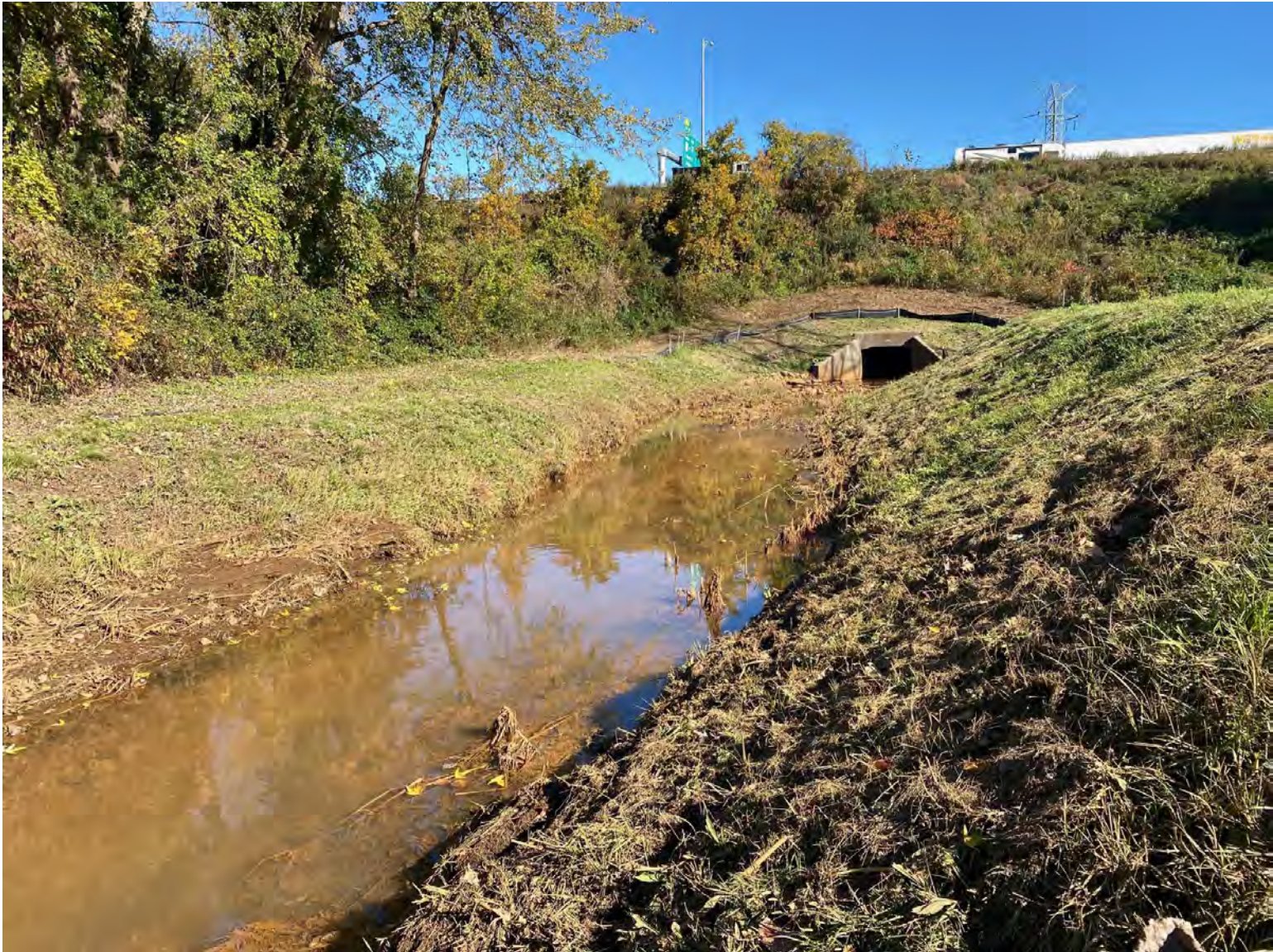
UPSTREAM END OF WESTERNMOST DITCH LOCATED BETWEEN ROUTE 9 AND I-91. SHOWING CULVERT BELOW I-91 AND REMNANT FLOODPLAIN TO THE LEFT.
