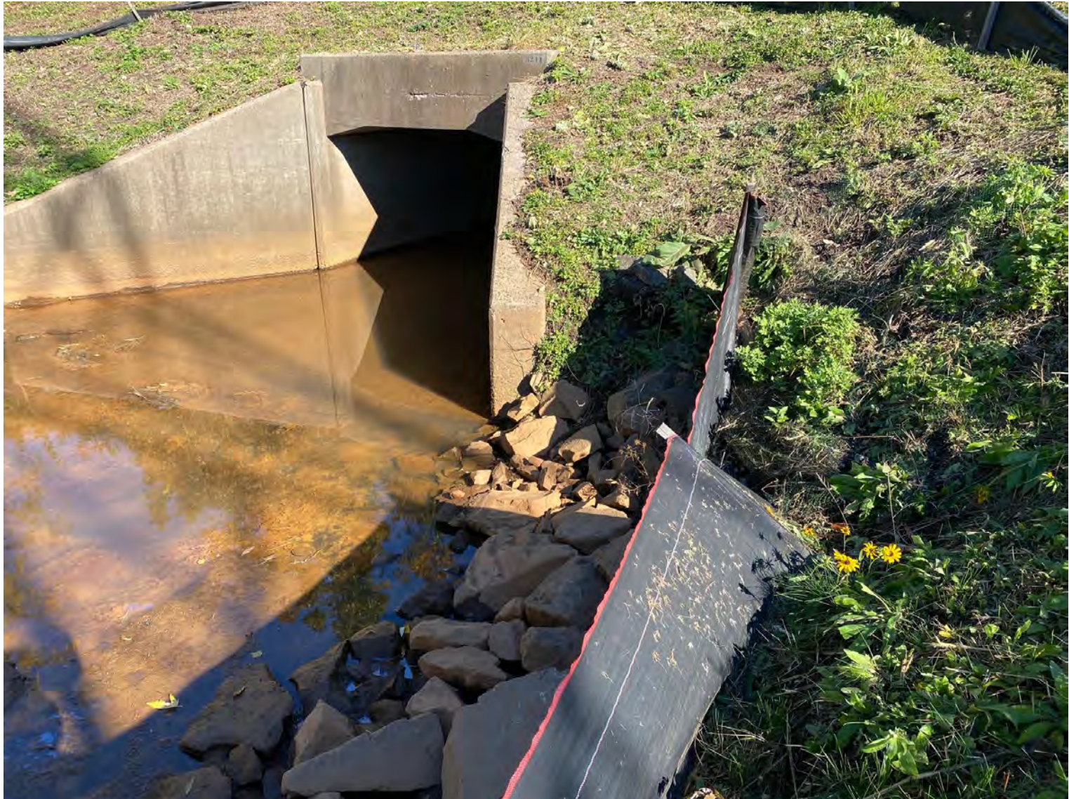
UPSTREAM END OF WESTERNMOST DITCH LOCATED BETWEEN ROUTE 9 AND I-91. SHOWING CULVERT BELOW I-91.
