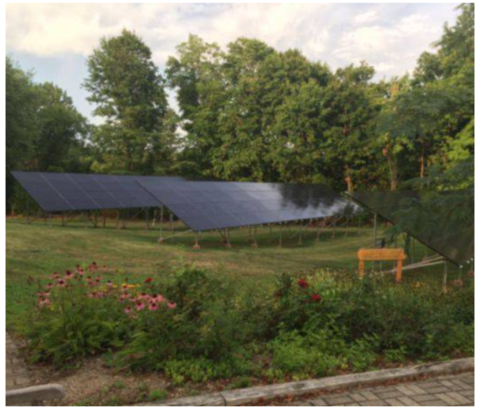
Figure G. Freestanding Solar. These freestanding solar panels, on the campus of a Hartford school, are well-screened by the landscape and fit nicely in the campus setting. (Photo courtesy S. Bronin.)
