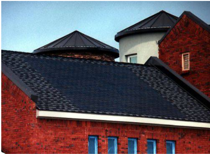
Figure E. Solar Shingles on a Pitched Roof. These solar shingles are designed to look like conventional asphalt shingles, matching them in size and color. (Photo courtesy National Alliance of Preservation Commissions.)
