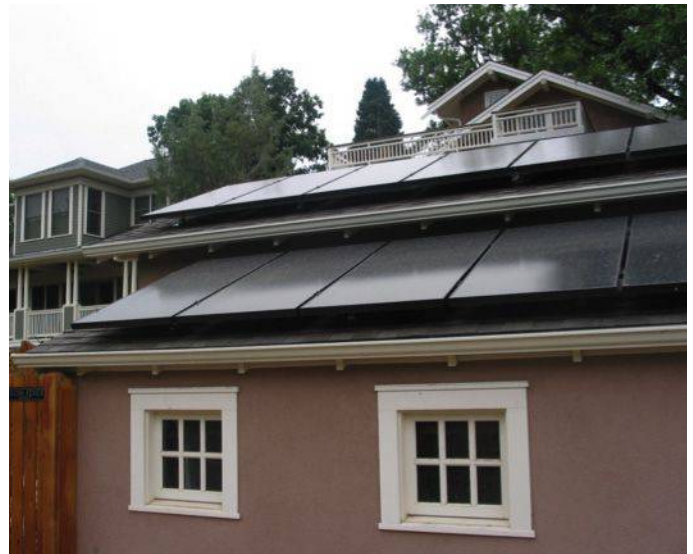
Figure F. Solar Panels on an Accessory Building. Solar panels placed on an accessory structure not visible from the public right of way should still follow the slope of the roof and have a low profile. (Photo courtesy National Alliance of Preservation Commissions.)
